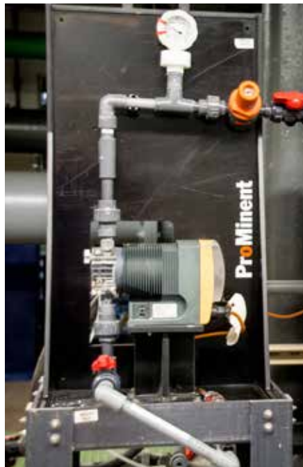
With the package feed systems, sensor technology, controllers and metering pumps form a unit that, along with the necessary storage tanks, were supplied to the authority as a “plug-and-play” solution. The customer-specific modular systems were tested by ProMinent and delivered to the plant on skids.
