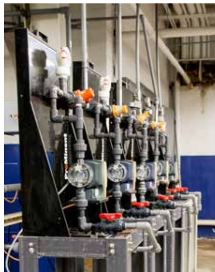
For many older facility's, such as the original side of the Shaler Water Treatment Plant, engineered modular systems can provide significant performance gains.
