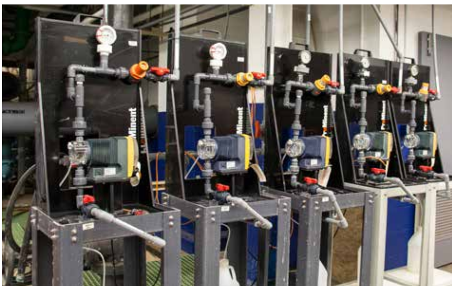
The Shaler Water Treatment Plant's gas chlorination equipment and pressurized gas cylinders were removed from the site. In their place, five fully integrated package disinfection systems, designed and engineered by ProMinent Fluid Controls, Inc, were delivered and quickly
