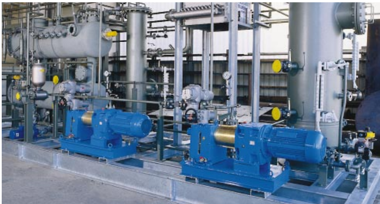
ORLITA® pumps (MfS 600/44 with electric stroke adjustment) in a glycol regeneration plant.
